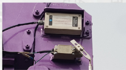
Overwinding Prevention System
